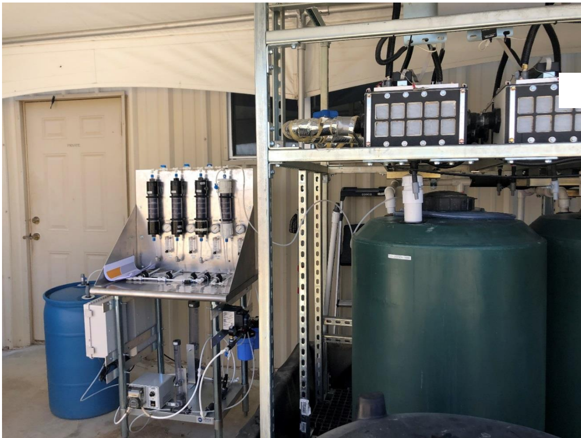
Figure 4: Aquacycl BETT™ and BioLargo AOS installed at Joshua Tree Brewery.
